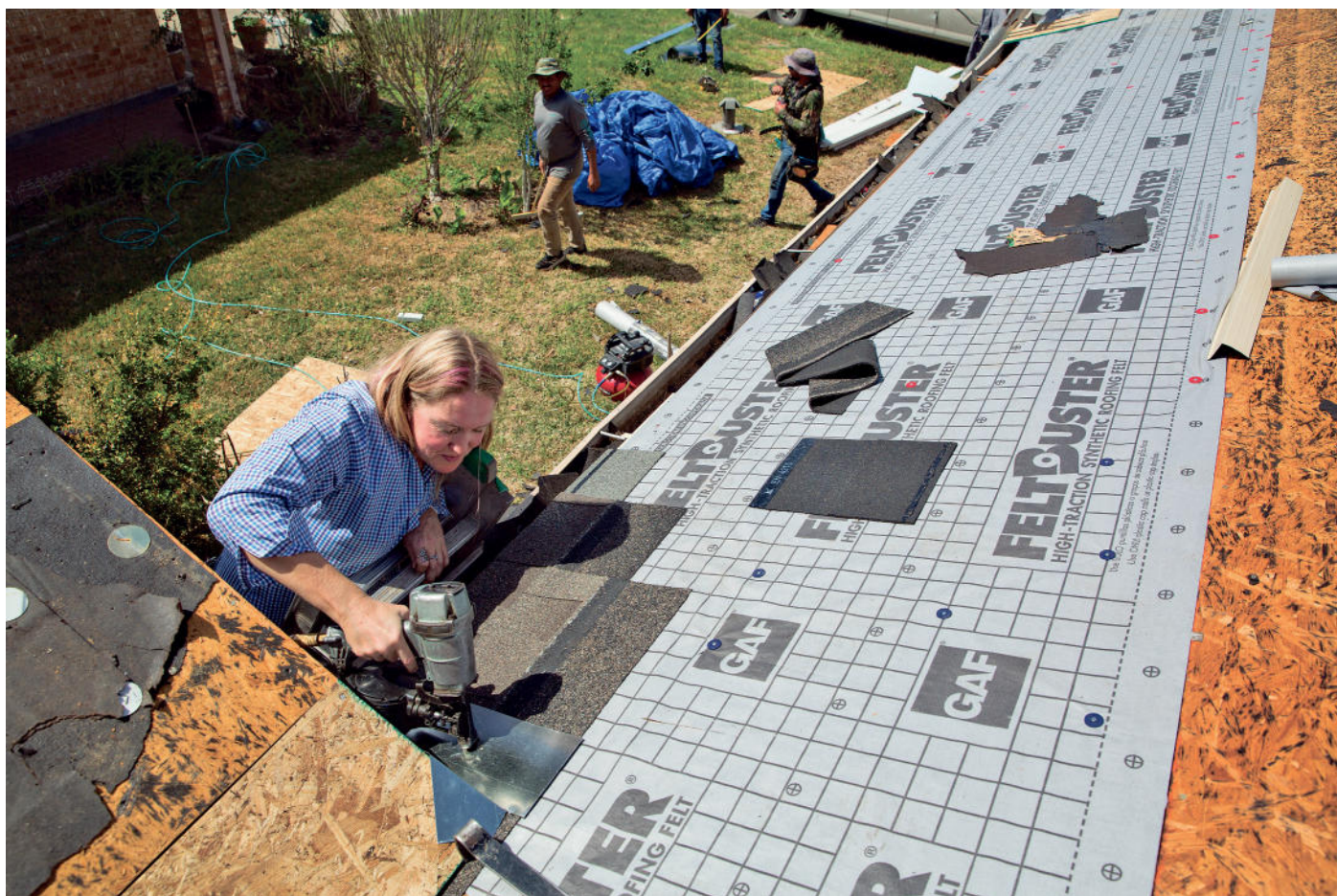
Ami Feller works on a customer's roof in New Braunfels on Tuesday, March 23, 2021. MIKALA COMPTON | Herald-Zeitung
