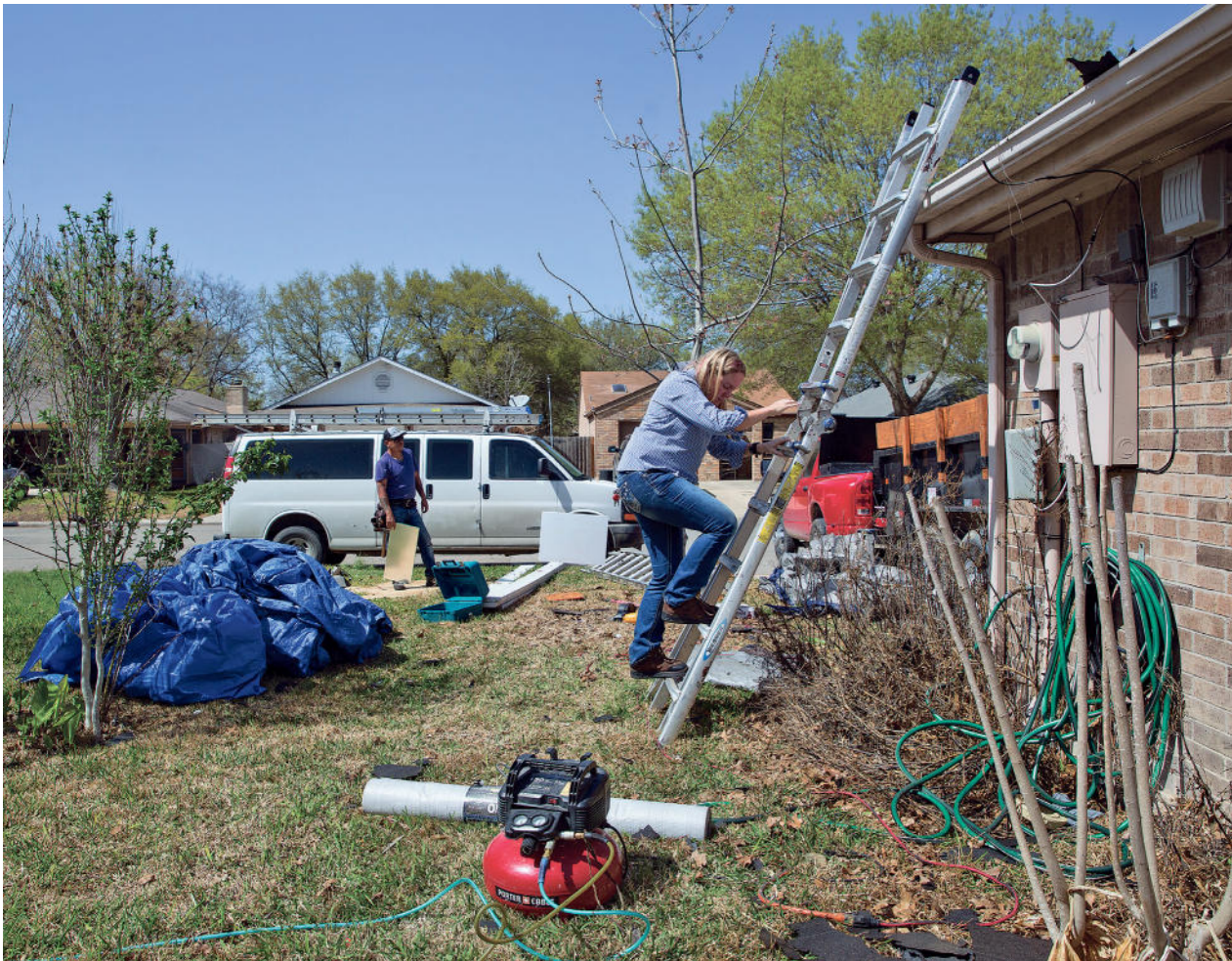
Ami Feller works on a customer's roof in New Braunfels on Tuesday, March 23, 2021. MIKALA COMPTON | Herald-Zeitung
